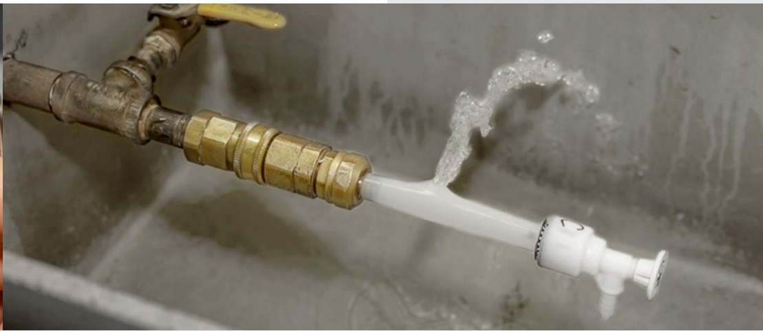
Daily hydrostatic testing. PEX pipe fails during test. ACCOR valve remains attached.
